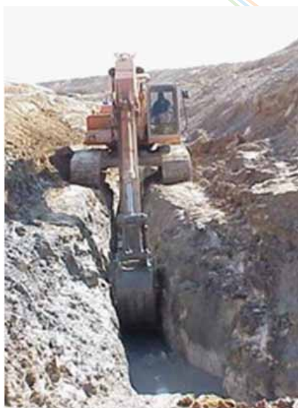
Figure 6: Drainage system installed along the local groundwater stream paths for the removal of hazardous pollutants from the Sechor-Besor aquifer
